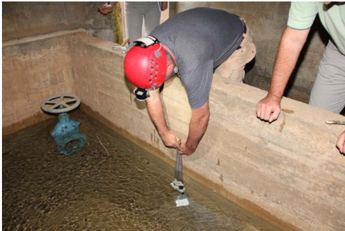
Installation of divers for measurement of water level, electrical conductivity, and temperature at the Kajža spring.
